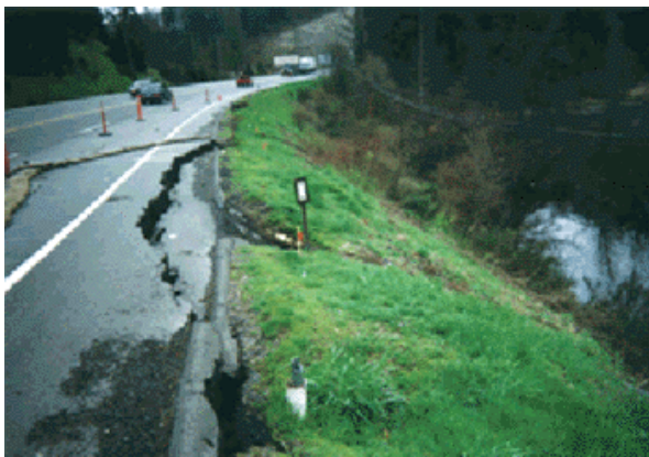
Figure 1 - Road Section Before Repair
